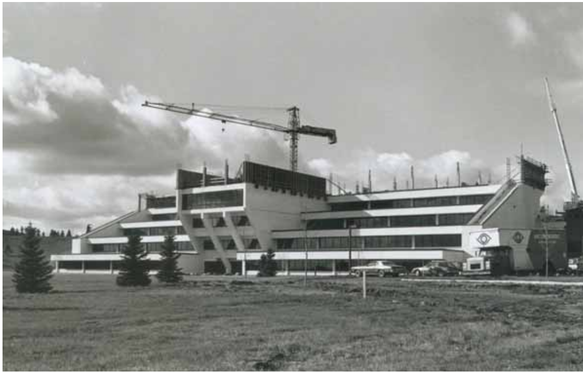
Submitted photo | Basin Electric Power Cooperative The construction of the Basin Electric Power Cooperative headquarters building in Bismarck in 1976.
