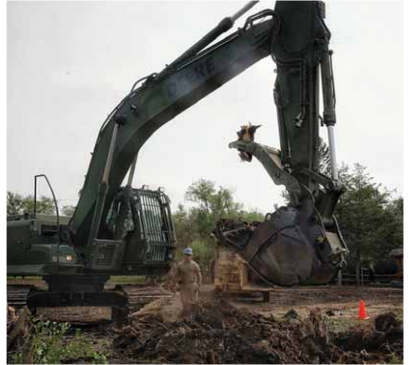
Sgt. Jessie Schuler, 188th Engineer Company, operates an excavator to remove tree stumps at Triangle Y Camp near Garrison, N.D. on Aug. 9. The Army Guard engineers worked on this Civil-Military Community project during their annual training period Aug. 1-15.
