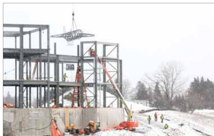
The B-52 "climber" was put in place at the Magic City Discovery Center in Minot! The Discovery Center was made possible due to a Defense Community Infrastructure Project grant. This was a combined effort between The City of Minot and Minot Air Force Base!
