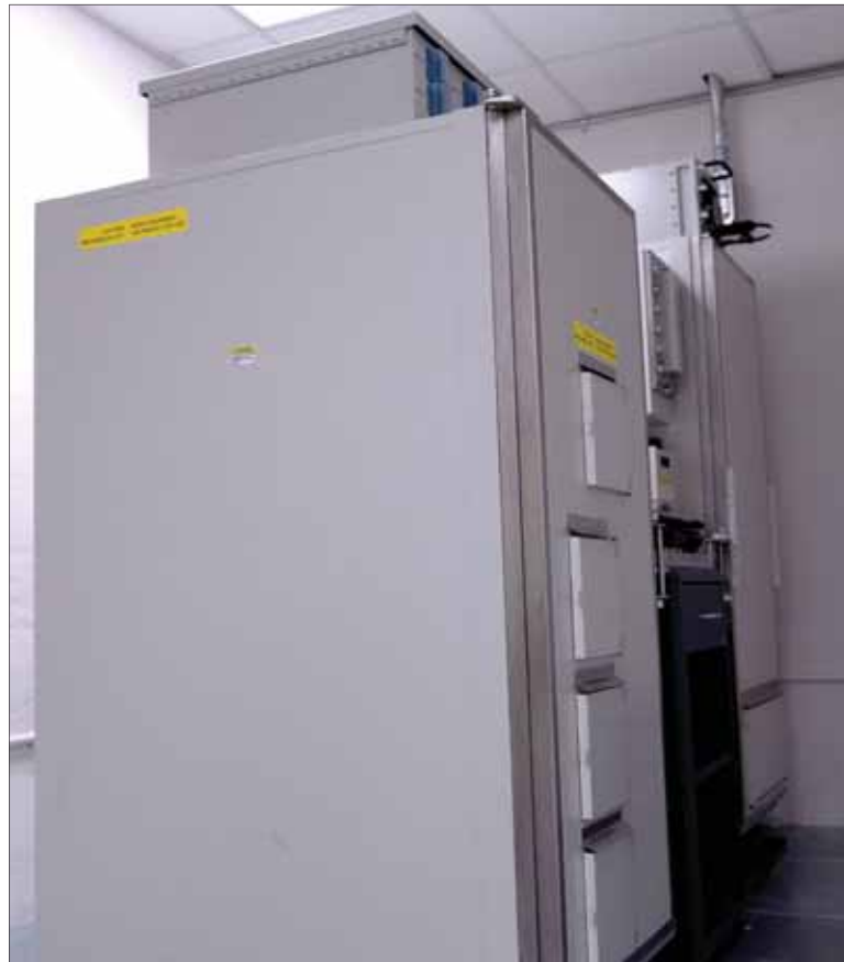
Recently installed Global Aircrew Strategic Network Terminal equipment powers up in the command post at Barksdale Air Force Base, Louisiana, Jan. 13, 2021. This equipment is the first of its kind and the first to be installed at Barksdale.
