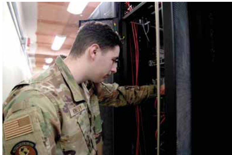
Senior Airman Nathan Kennedy, 608th Air Communications Squadron system administrator, inspects servers in the 608th ACOMS data center. An important part of his job is to ensure all systems are on and running 24/7 with the most current upgrades.
