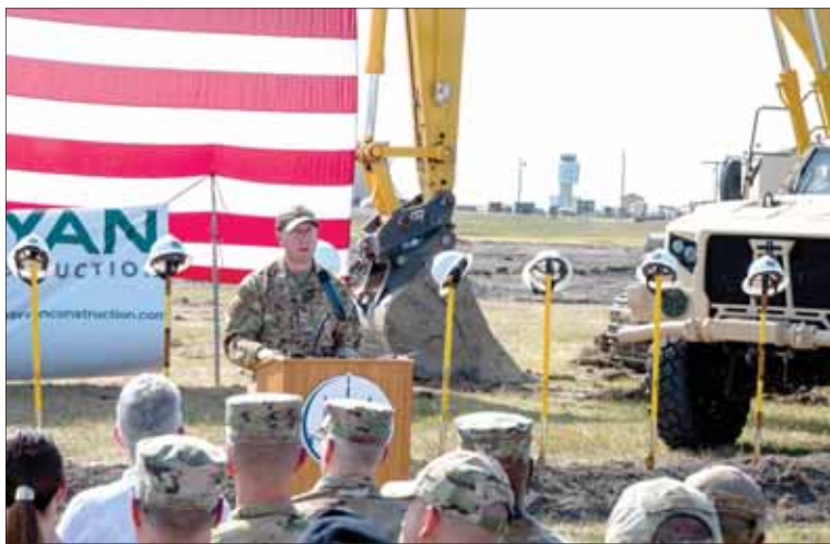
Col. Daniel Hoadley, 5th Bomb Wing commander, gives remarks at the groundbreaking ceremony for the 54th Helicopter Squadron's new facility Aug. 16, 2023, at Minot Air Force Base, North Dakota. The new facility will house the incoming MH-139 Grey Wolf, which will replace the current UH-1N Iroquois.
