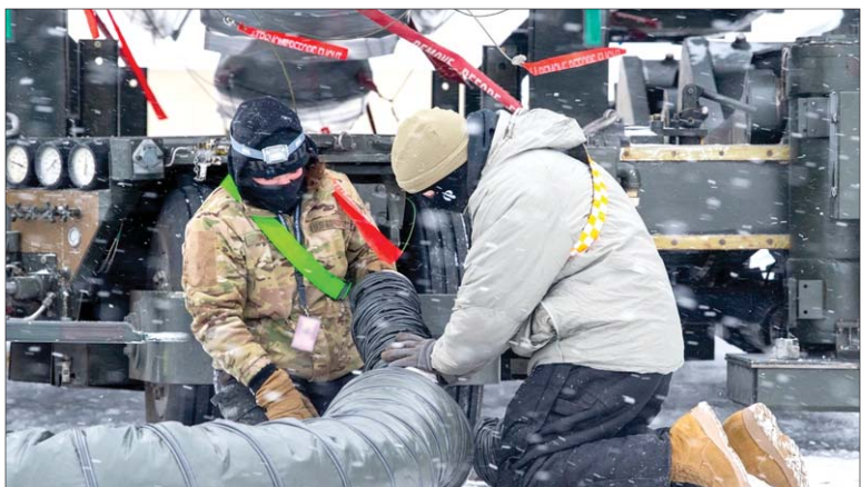
Airmen from the 2nd Aircraft Maintenance Squadron work on a flightline heater tube in support of Exercise Prairie Vigilance/Bayou Vigilance 24-2 at Minot Air Force Base, North Dakota, Jan. 7, 2024. The exercise enhances readiness while ensuring that associated strategic assets are safe, secure, and effective.
