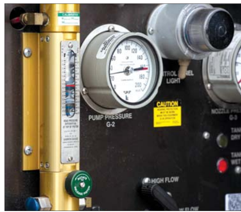
A fuels control panel is displayed on an R-11 fuel truck at Minot Air Force Base, North Dakota, March 7, 2024. The gauges indicate to equipment operators the fuels distribution equipment is functioning correctly and safely.
