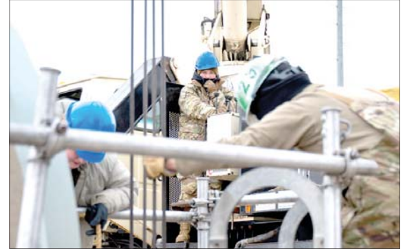
Senior Airman Audrey Smith (center), a 91st Missile Maintenance Squadron electro-mechanical team technician, uses a crane to lower a replacement battery into a launch facility near Minot Air Force Base, North Dakota, April 2, 2026. The Minuteman III intercontinental ballistic system dates back to the 1960s and its longevity demands consistent upkeep.
