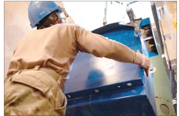
Senior Airman Benjamin Delaney, a 91st Missile Maintenance Squadron electro-mechanical technician, lowers a battery into a launch facility near Minot Air Force Base, North Dakota, April 2, 2026. Despite the inherent risks of working with high-voltage systems and heavy mechanical equipment, safety remains a constant priority for the EMT.
