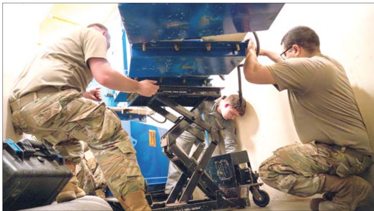
Airmen from the 91st Missile Maintenance Squadron's electro-mechanical team (EMT) replace one of the many batteries in a launch facility near Minot Air Force Base, North Dakota, April 2, 2026. Many of EMT's procedures fall under strict nuclear surety guidelines, which demand step-by-step adherence without deviation.
