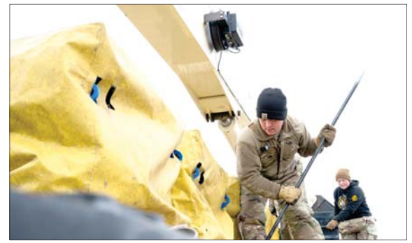
Senior Airman Andrew Constancio, a 91st Missile Maintenance Squadron electro-mechanical team chief, pries loose chain links holding replacement batteries for a launch facility near Minot Air Force Base, North Dakota, April 2, 2026. These Airmen play a vital role in sustaining the old, yet still formidable Minuteman III intercontinental ballistic missile system.
